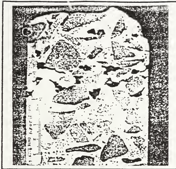
Figure 2.14 Honeycombing within concrete (Reference 4)
